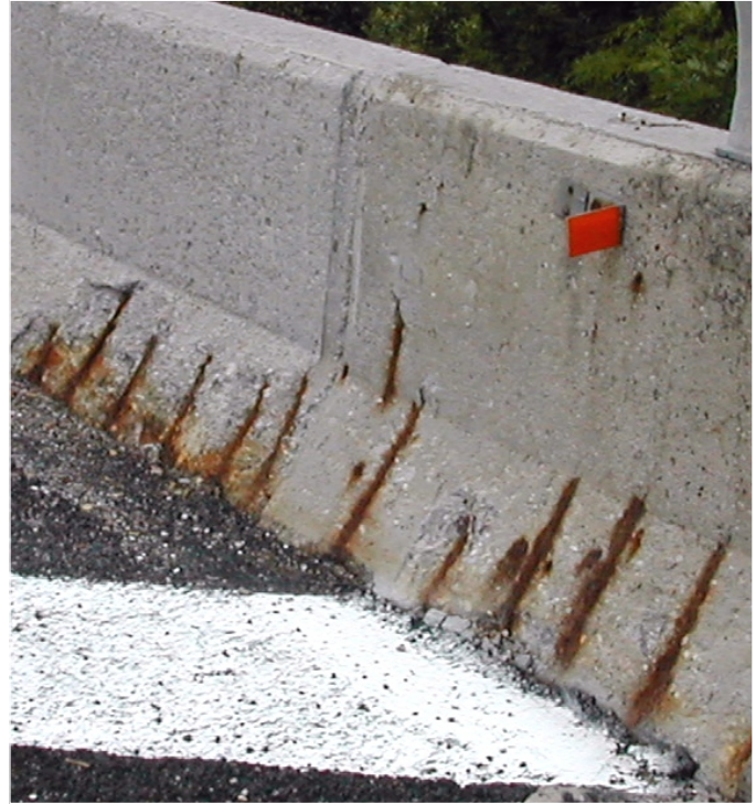
Exposed rebars due to carbonation effects
